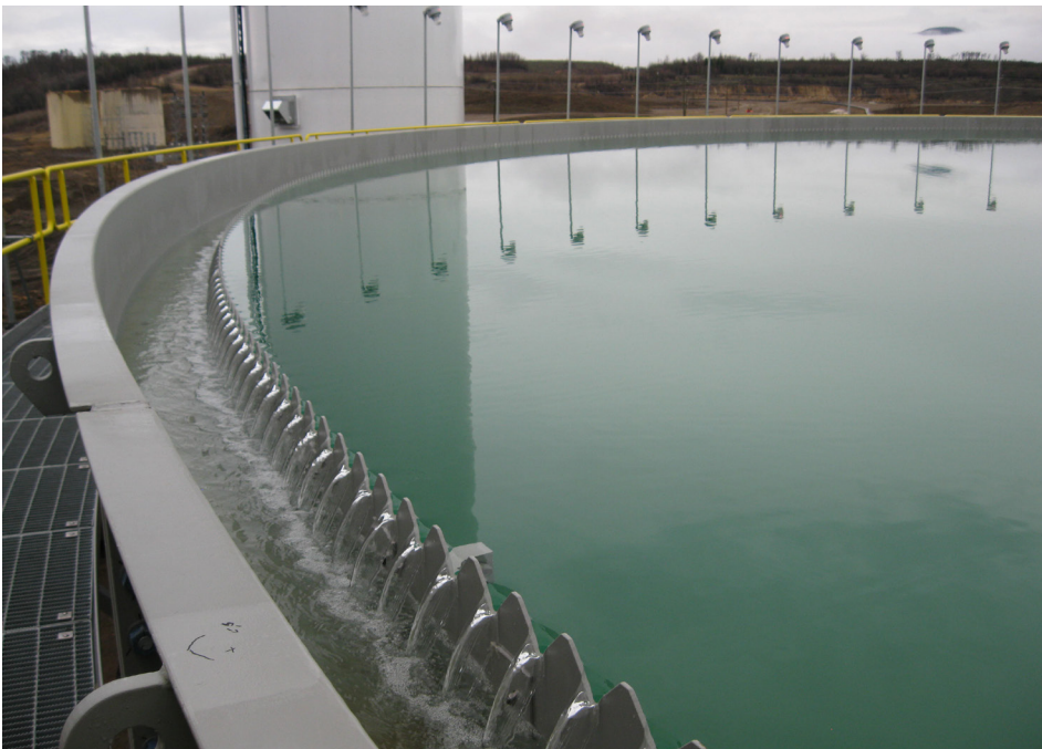
An FLS clarifier providing amazing overflow clarity
