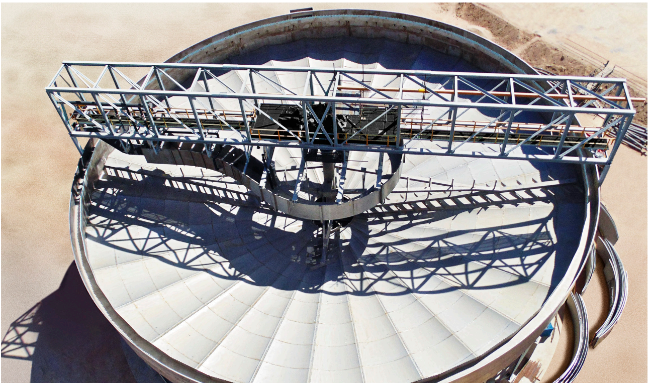
FLS high-rate thickener prior to being commissioned
